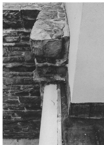
Fig. 8. The existing EPDM membrane is secured with "hit"-fastened termination bars. Both the sealant along their perimeter and the gaskets at the "hit" anchors have failed. The complicated nature of waterproofing diverse construction materials — stone and concrete — where they abut is self-evident. Photograph by WASA.
