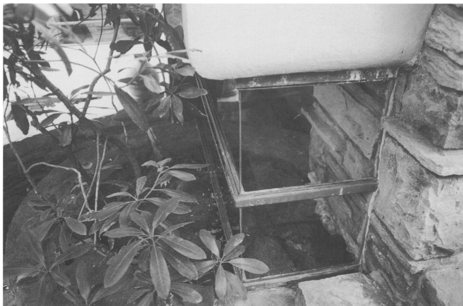
Fig. 6. Fixed panes of glass sometimes terminate directly into stone walls. These lack waterproofing details of a standard frame. In addition, corrosion occurs at window heads as a result of the rounded edge of the concrete soffits and the lack of metal drips at the main house's fixed windows. Photograph by WASA.
