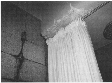
Fig. 9. Moisture infiltration in the main house's guest bathroom continues to damage both the plaster and cork-tile finish. Photograph by WASA.
