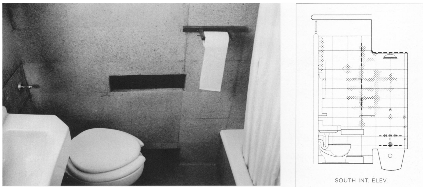
Fig. 7. Photograph and detail of drawing from the Existing Conditions Survey, showing the condition of the guest bathroom in the main house. Drawing by WASA.
