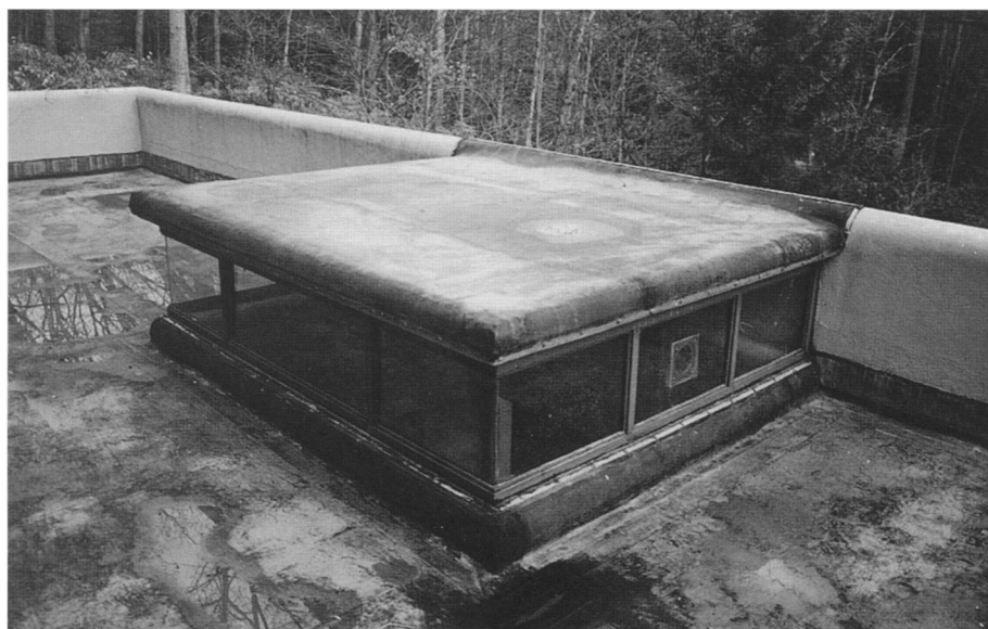
Fig. 10. The monitors are particularly difficult features to waterproof. This one is located over the guest-house bathroom and is responsible for substantial damage to the interior finishes. Photograph by WASA.
